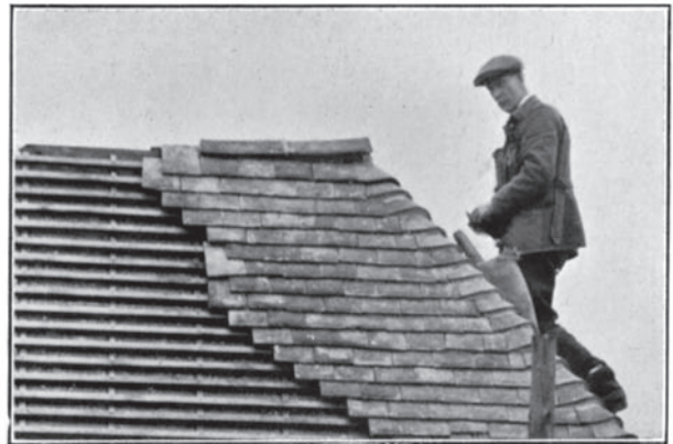
FIG. 21. Two faults are here illustrated. (1) The ridge tiles are not bedded down sufficiently closely. (2) The heading course of plain tiles and the hip tile of that course dip downwards instead of being tilted up slightly (as are those in the two courses below) to help the tilting of the end ridge tile.
