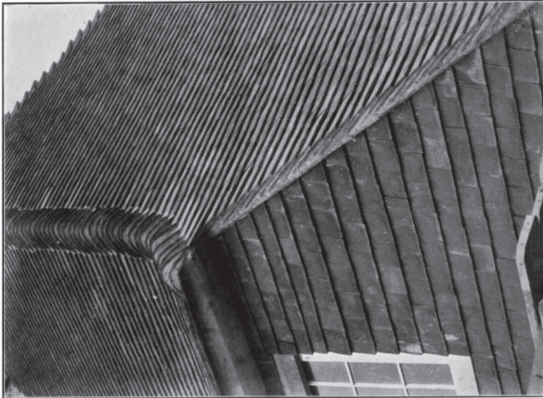
FIG. 12. (a) Right—and strong verge with undercloak tiles. (b) The board over the head of the window frame temporarily supports the heading course of wall tiles bedded in cement.
