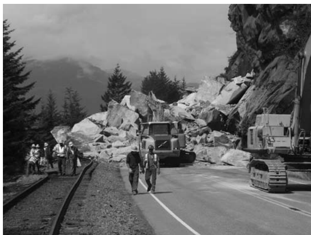
Fig. 1. Rockslide on the “Sea-to-Sky Highway” (Highway 99) north of Vancouver, British Columbia. This landslide interrupted traffic along a major transportation corridor connecting Vancouver and Whistler, site of the 2010 Winter Olympics. (Photo courtesy of Erik Eberhardt.)
