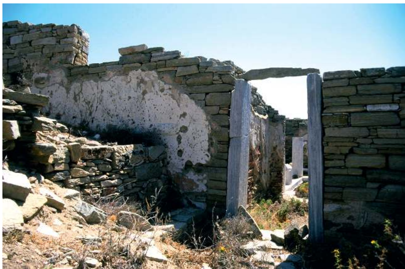
Figure 1.1 Exterior wall showing the remains of a plaster coating. Delos, Lake House. (Author's photograph, courtesy of the Ephorate of Antiquities of the Cyclades. The rights to the monument shown belong to the Hellenic Ministry of Culture and Sports (Law 3028/2002). Delos is under the supervision of the Ephorate of Antiquities of the Cyclades, Ministry of Culture and Sports.)
