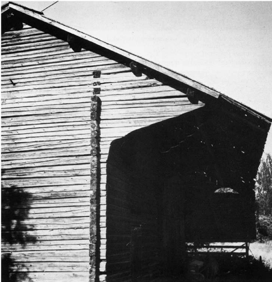
3 Modern farm building in Vöyri district, Finland, showing cantilevered support of overhanging roof.
