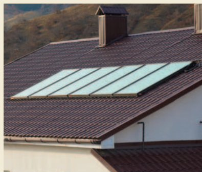
Photovoltaic solar panels
